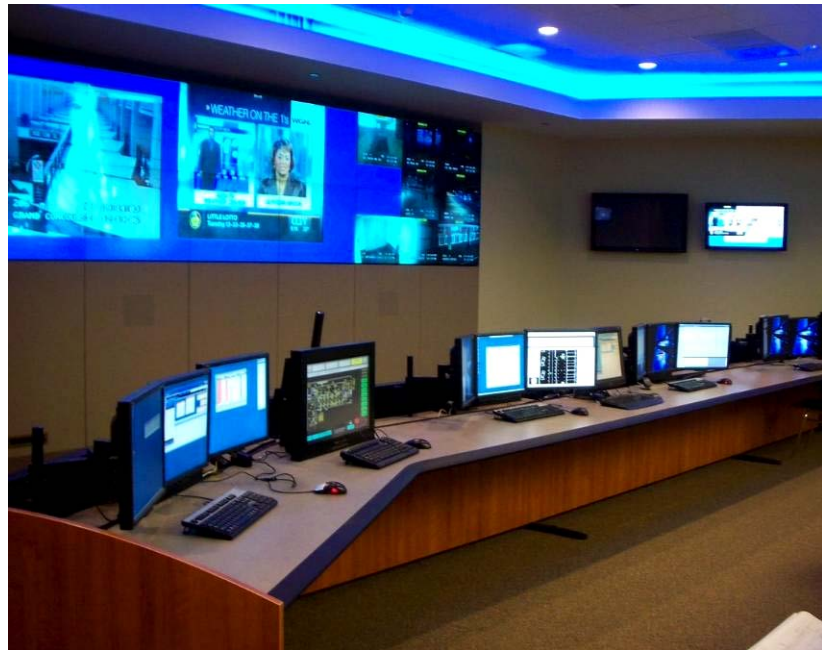
Figure 2: SDI Command Center design. No computers are housed in the Command Center; all equipment is now housed in Data Centers, where it is protected and secure. Desks are less cluttered, and all systems are now available at every workstation.
