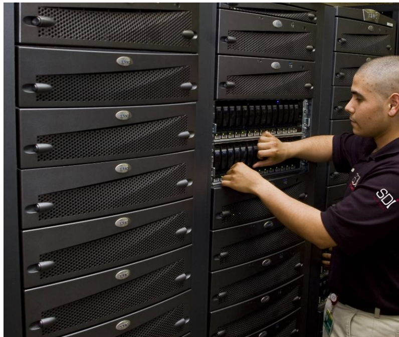
Figure 4: Storage Area Network at an SDI Airport Command Center client. Storage alone accounts for much of the square footage of today's Public Safety Data Centers. For example, this client retains video from 3,000 cameras for 15 days, requiring robust, multi-terabyte data storage.
