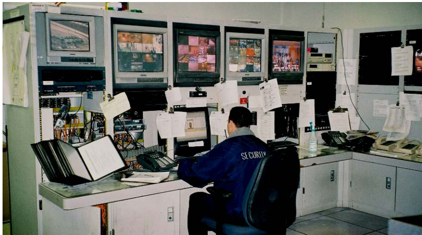
Figure 1: Existing console-based systems before SDI re-design. All equipment is housed in consoles. Frequent issues arise from damage to equipment, and operators must physically move from one system to another.
